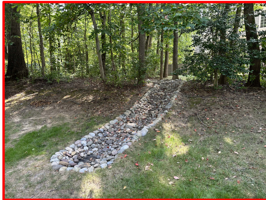
IMG_0527.jpg Channel 6A (Not Shown on 2009 Plan) 4' avg. width, 2-6" avg. stone size
